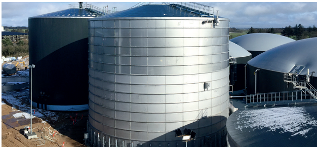
Drei zentralgerührte Fermenter im Bau Three continuous stirred tank reactors during construction
