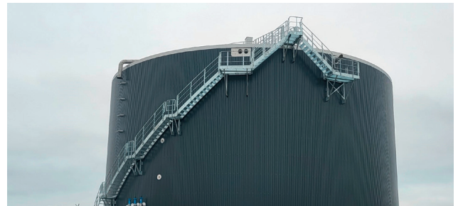
Tankmanteltreppe Tank Staircase
